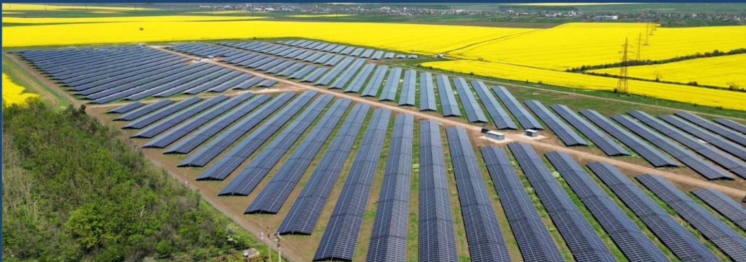
Premier Energy's 26 MW Da Vinci solar park development with a battery storage capacity of 10 MWh in Nanov, Teleorman county, Romania .
