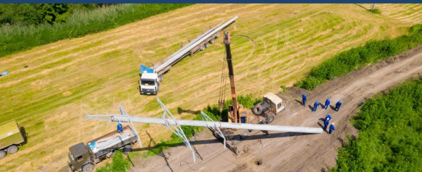
Premier Energy's 110kV overhead power line (LEA) CET-2, Codru substation, Chisinau, Republic of Moldova.
